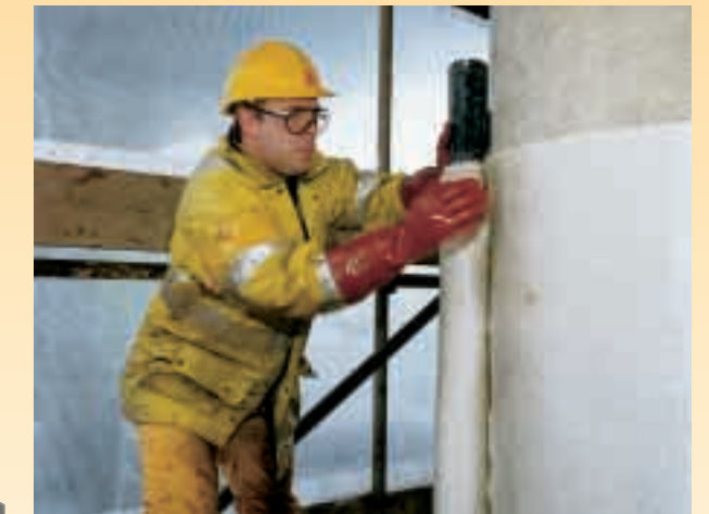
Application of SikaWrap® Fabric System for impact resistance on a bridge column
